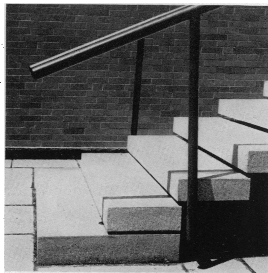
Detail of stairway to sculpture court. Granite slabs rest on inclined reinforced concrete beams; the two lower slabs rest on the ground.
